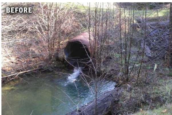
The undersized and degraded culvert at the mouth of Wolfe Creek blocked fish passage to upstream habitat for wild populations of steelhead and Chinook and Coho salmon.
