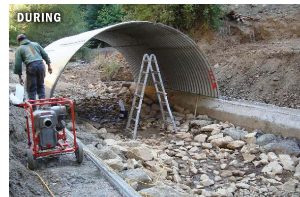
The undersized culvert was replaced with a bottomless culvert arch. The natural stream bottom improved conditions for the steelhead and salmon populations in the Mattole River watershed.
