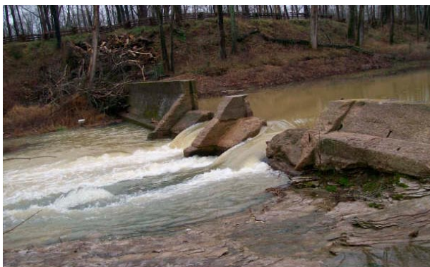
The Sandy Hook Dam on Big Bigby Creek prevented fish passage in six miles of fisheries habitat. The dam altered stream flow and fish passage as well as negatively affected the in-stream fisheries habitat.
